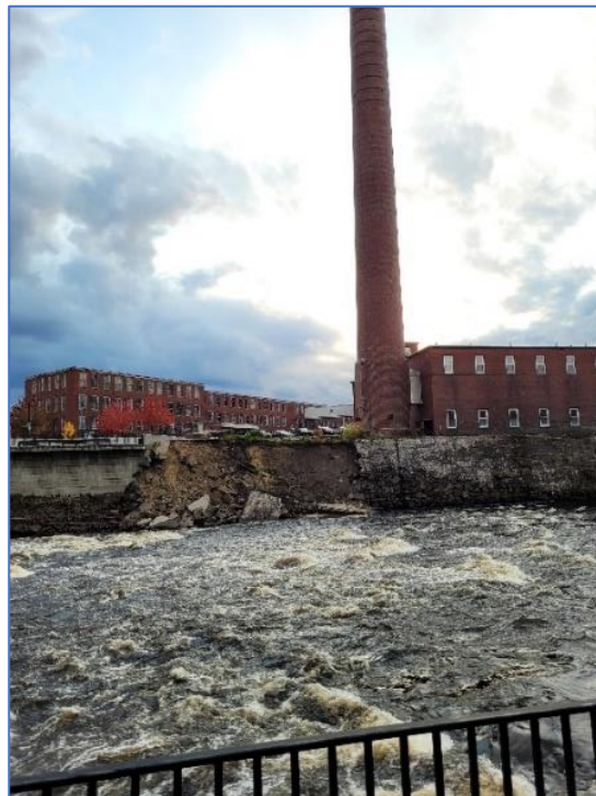
Figure 8 A section of the stone riprap along the Saco River in the Biddeford Mill District was damaged during an extreme precipitation event and subsequent high River flows in late October 2021. Credit: A. Sherwin
