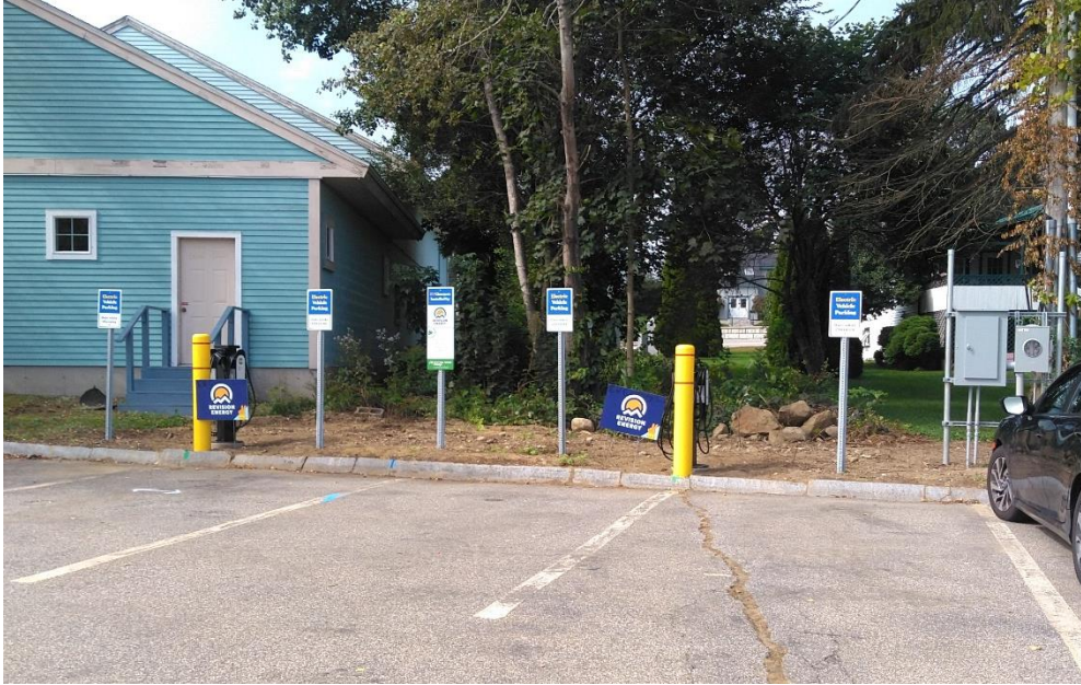
FIGURE 10. PUBLIC EV CHARGING STATIONS AT KITTERY TOWN HALL.
